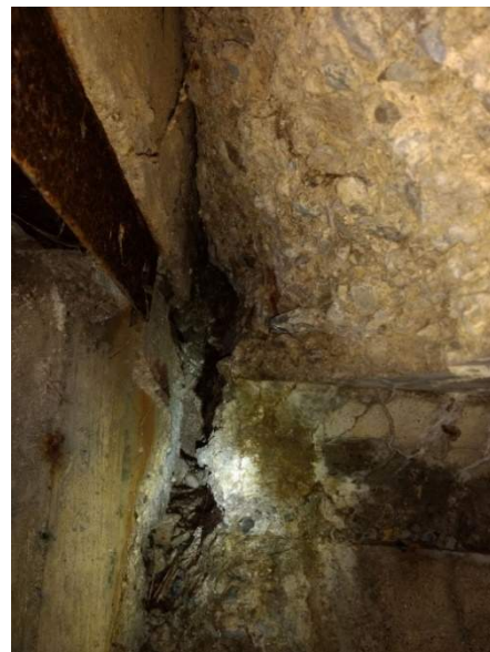
Figure 2: Bishop Ck Culvert WB travel edge
